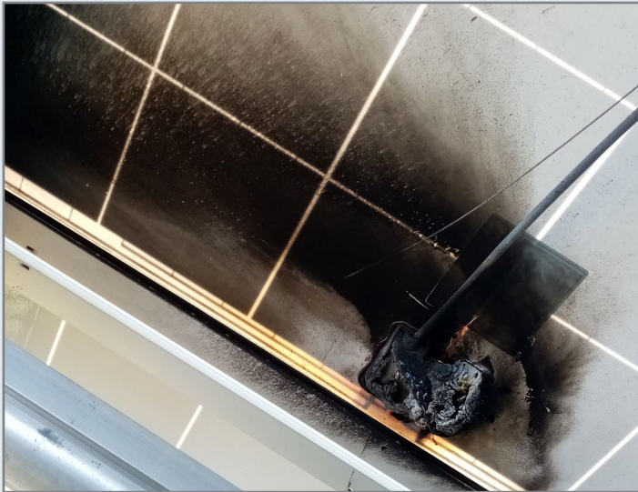
The image above shows a PV module at the project site with a junction box that melted due to electrical arcing.
